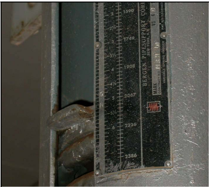
Figure 5. An exemplar variable support hanger scale showing travel and supporting load.
