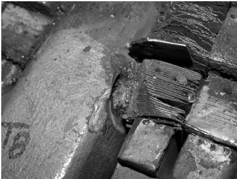
Failure due to Loose Step Iron
