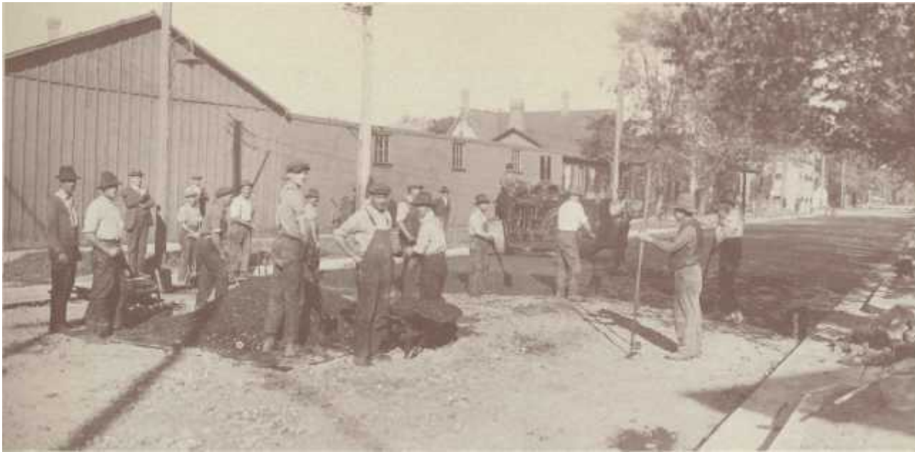
Another view of paving - - the hard way - - on Marl- borough Street in the block between West and Market.
