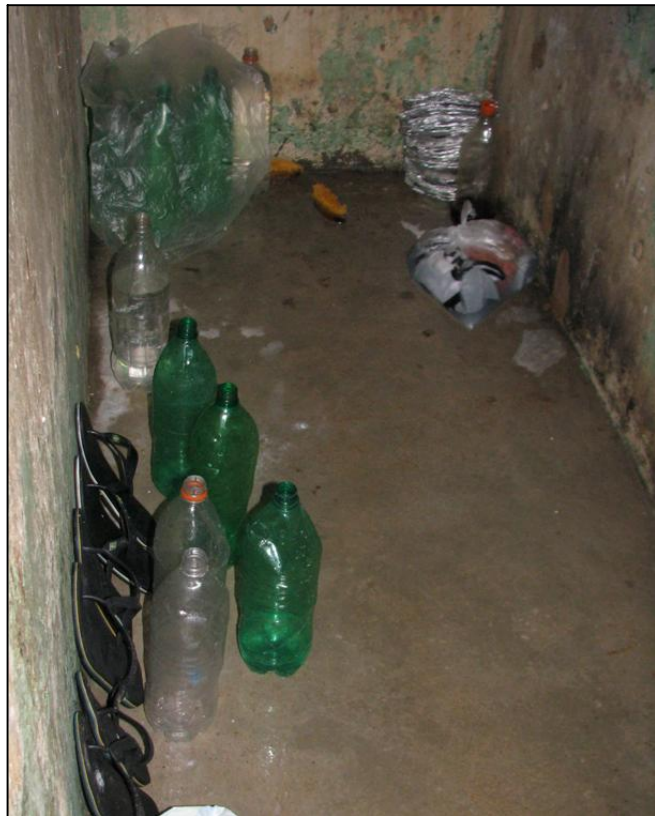
Photo 7: The cells are in very bad shape and do not have adequate hygienic provisions. (Photo source: LAPL)
