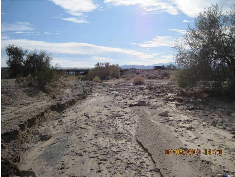
Figure 21. Incised and scoured channel immediately downstream of I10. Bank detail shown in next photo.
