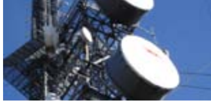
Service tower, Truskmore Mountain, Co. Sligo
