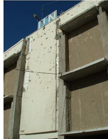
Figure 6: Aida Girls School in the West Bank after crossfire damage
