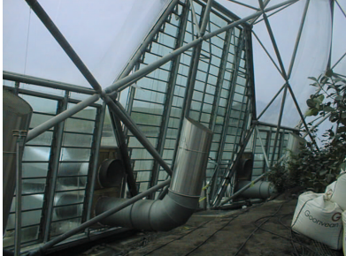
Fig. 13 Vents and heating
