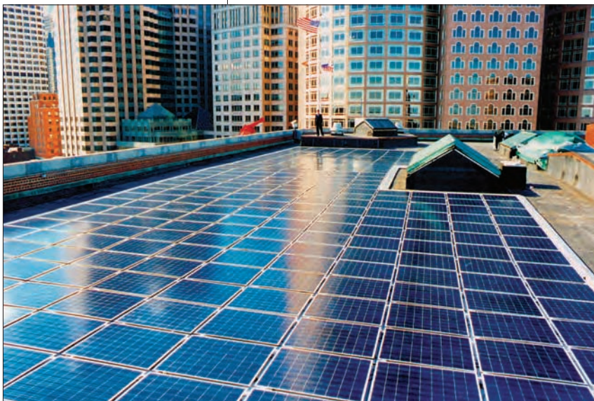
PV panels atop U.S. Coast Guard Building, Boston, Massachusetts.
