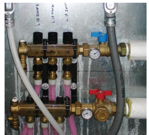
PEX piping and valves are visible inside wall cabinets to allow explanations for how the system works to visitors
