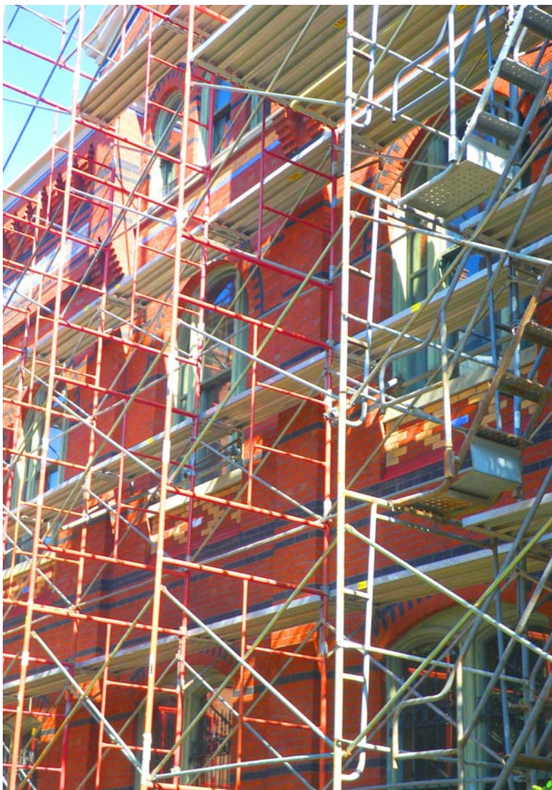
Scaffolding on the Arts and Industries Building for masonry repair funded by the American Recovery and Reinvestment Act Image credit: Steven Townsend
