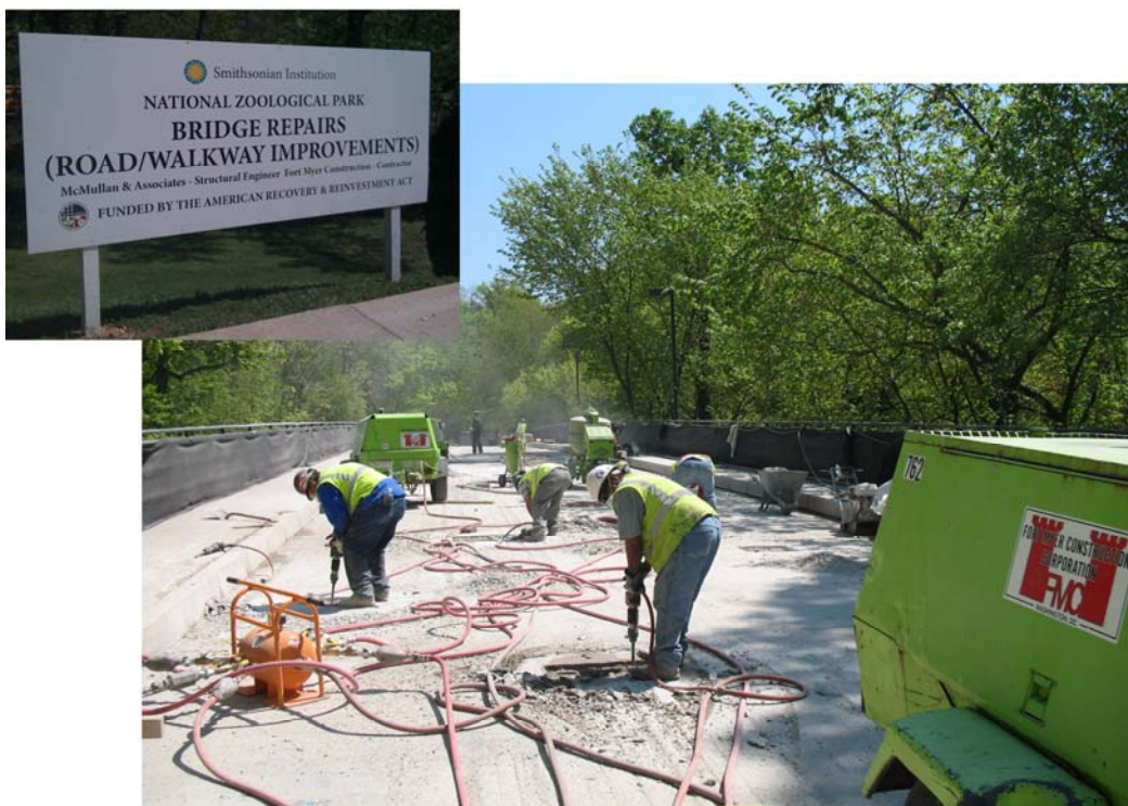
Workers repairing the Harvard Street bridge connecting the National Zoological Park to Adams Mill Road, NW, a project funded by the American Recovery and Reinvestment Act.
