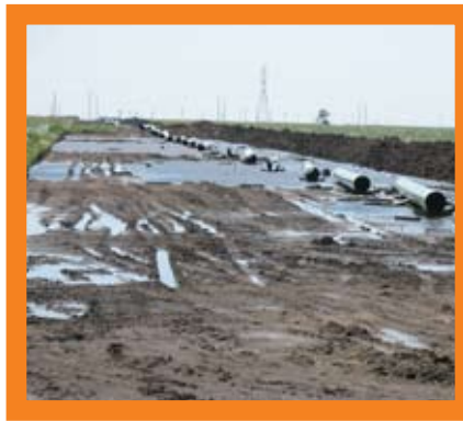
The Keystone tar sands pipeline being laid across a landowners property. The earthen berm, intended to limit water along the pipeline path, is drowning the property owner's crops.
