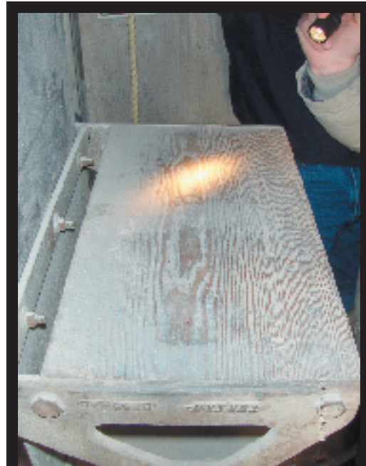
The worn down wooden step on the belt operated man lift.
