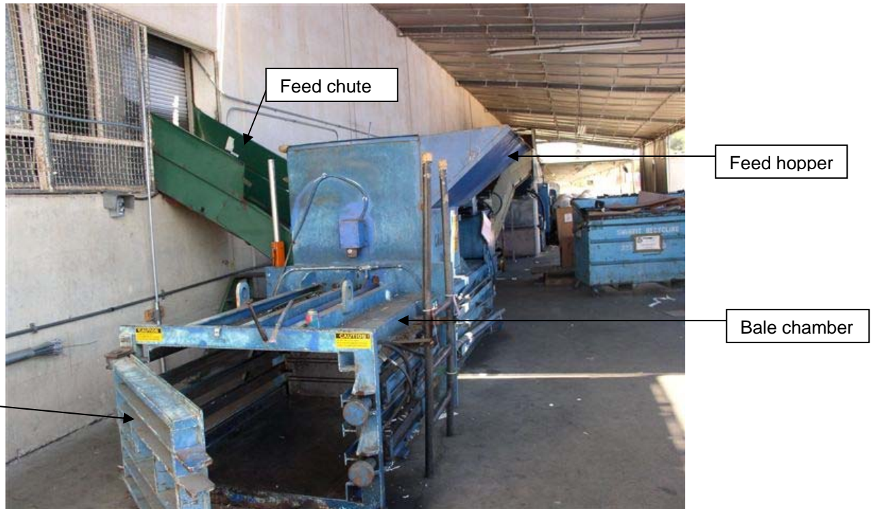
Exhibit 3. The cardboard baler showing the feed chute and chamber where the recycled bales of cardboard were formed.
