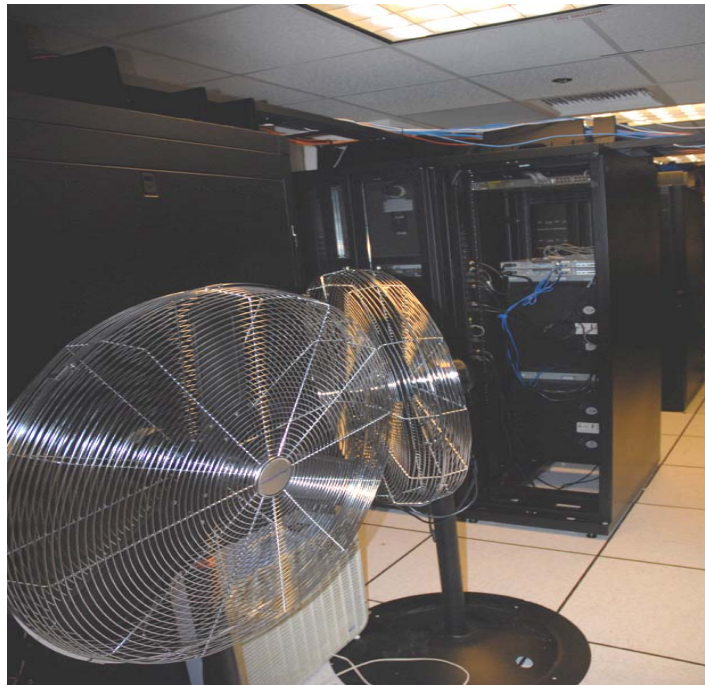
Figure 2. Fans Cooling Server Equipment
